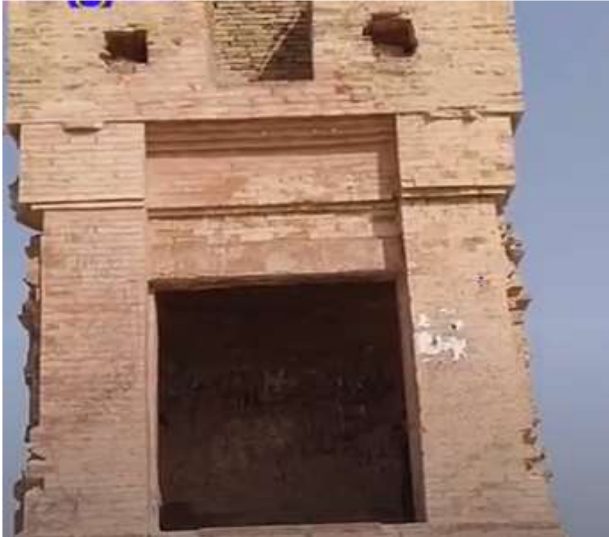
Fig.9. The doorway opening from the west (10' x 6' 2") is restored under Vats' supervision.
